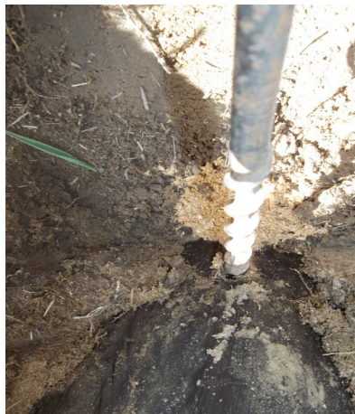
Looking down as a hole is bored into the pole base, checking internal integrity.
